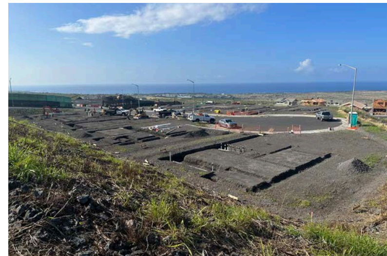
Footings of house excavated, underground plumbing all roughed in, awaiting termite treatment and concrete pour at Laiopua Village 4 Phase 1 - Akau, Increment 2
