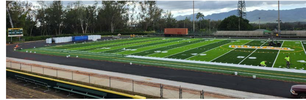
Leilehua HS field project work advances, as shown from the progress from December to February
