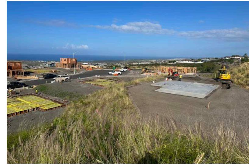
View of the homes being framed, slabs prepped for concrete pour, and one slab completed and lot being dessed from around the edges at Laiopua Village 4 Phase 1 - Akau, Increment 2
