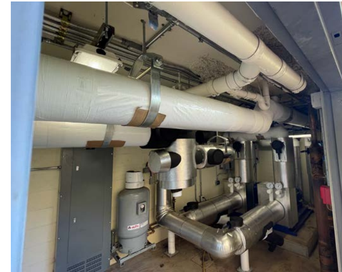
Building 502 - Chilled Water Pump Room
