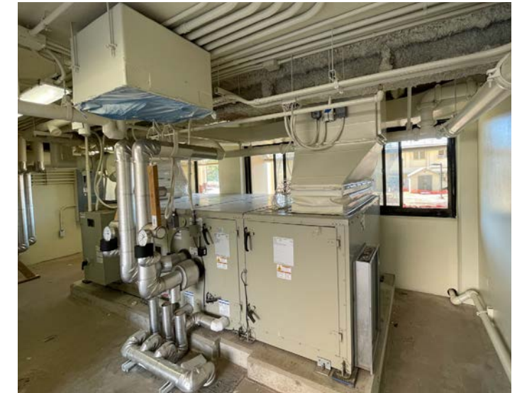
Building 502 - Mechanical Room with DOAS Unit
