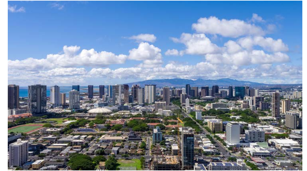
Drone shot taken by the IT Team from the future 44th floor of Liona Tower at The Park on Keeaumoku currently being constructed by Nan, Inc.
