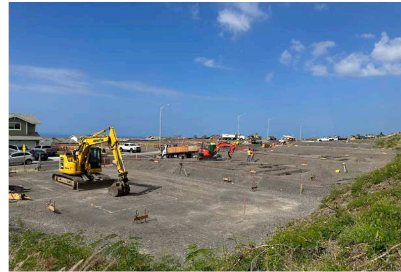
Crews excavating house footings and underground plumbing at Laiopua Village 4 Phase 1 - Akau, Increment 2
