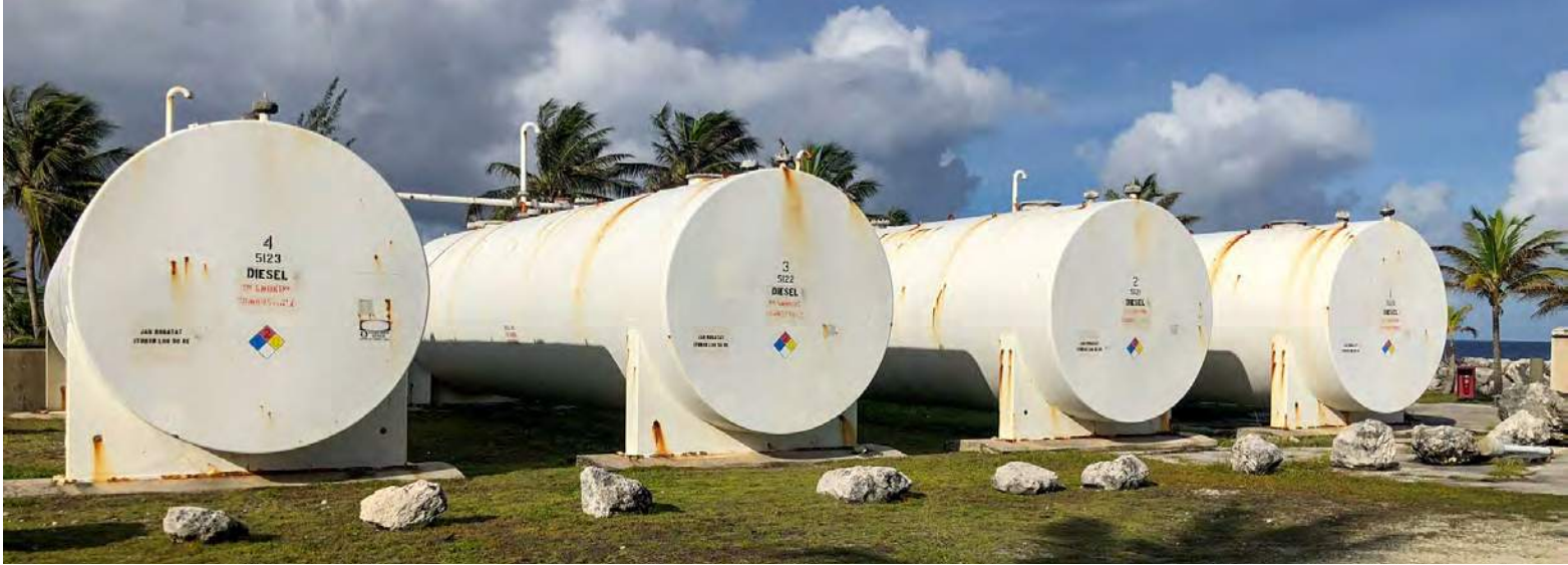
Meck Island fuel tanks
