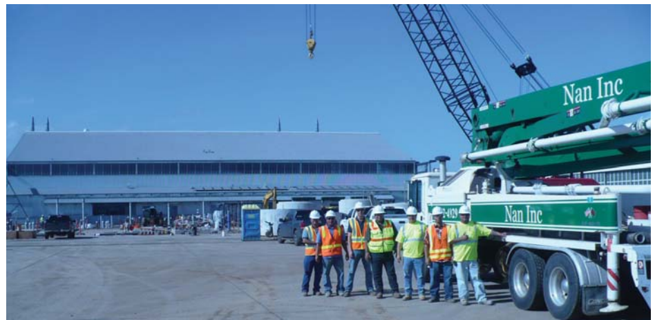
Team NOAA fronting the project facility and the company concrete pump truck
