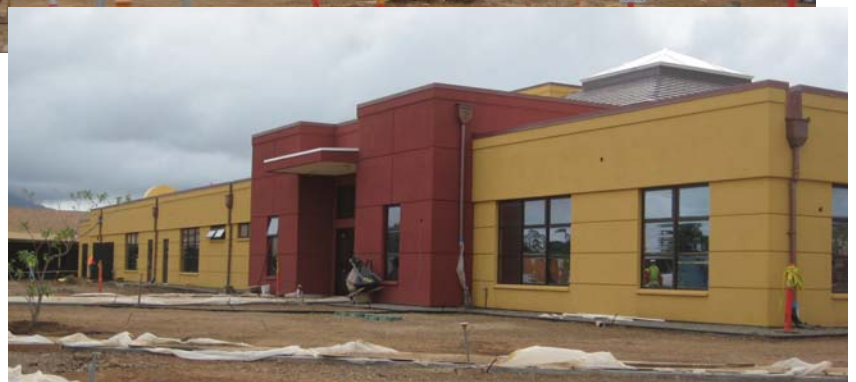
Progress Views of the Main Entrance and Front of the Youth Center
