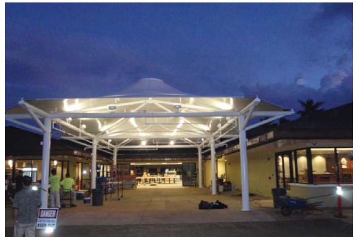
New tension structure for Klipper Club House renovation, designed and installed by Tropical J's
