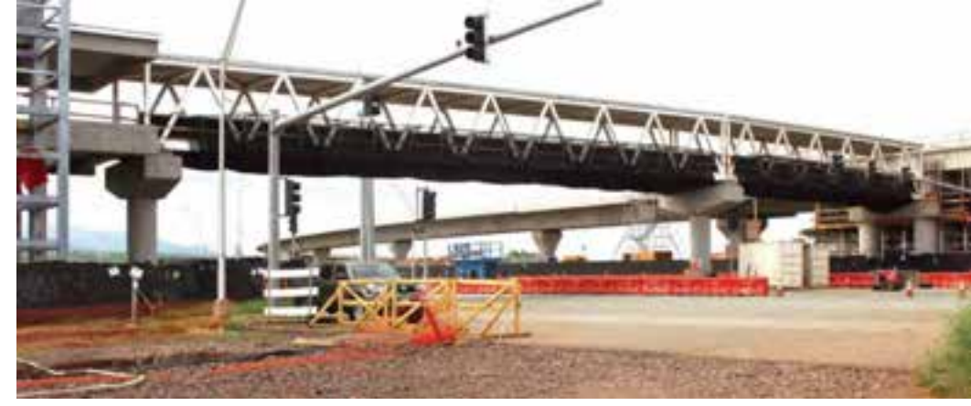
Photos, from the top: Pedestrian bridge at Keoneae (U.H. West Oahu) rail station shortly after the second massive span was installed over Kualakai Parkway; Aerial view of Road "B" and Temporary Park and Ride construction site at U.H. West Oahu; Governor David Ige joins Nan, Inc. construction team for photo at East Kapolei Middle School groundbreaking ceremony; 2.5 million-gallon water tank under construction in Kunia for the Hoopili Off-Site Water System
