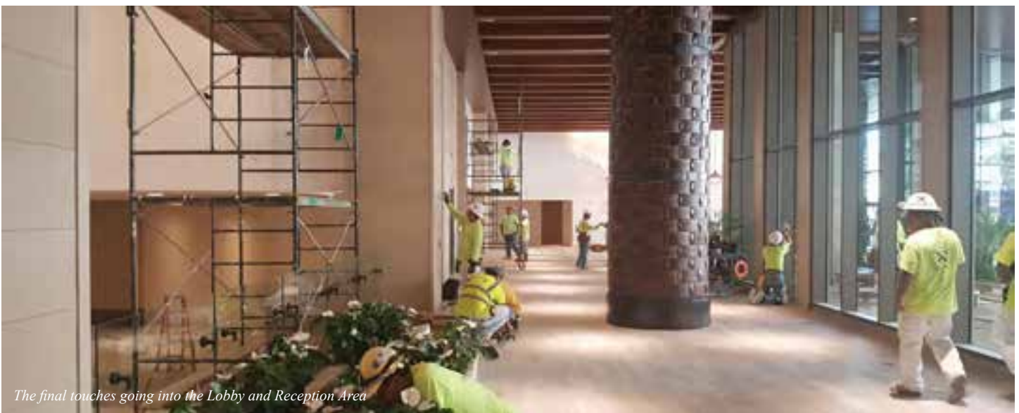
The ongoing installation of the millwork and shelving at the Bar in the Lobby Lounge
